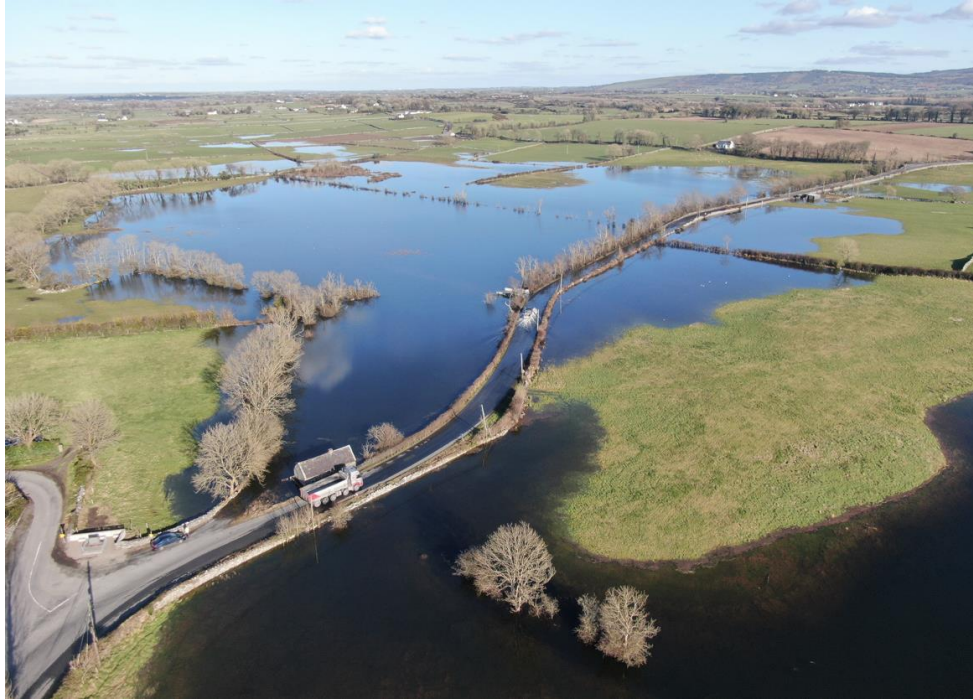
Receding Flood Levels of March 2020. The road flooded over a total length of 400m to a maximum depth of 500mm
