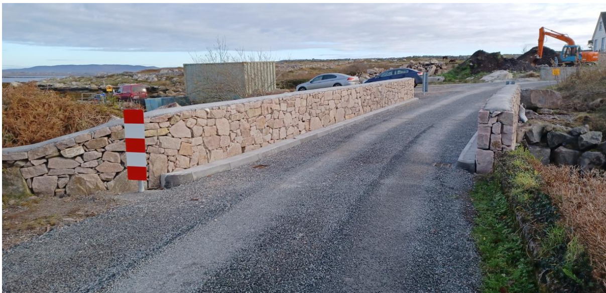
Pictures above show bridge at Sruthaun Buí, Lettermore before and after works undertaken
