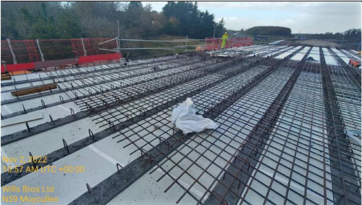
Installation of Steel Reinforcement for ST07 Lough Kip River Bridge Deck Pour
