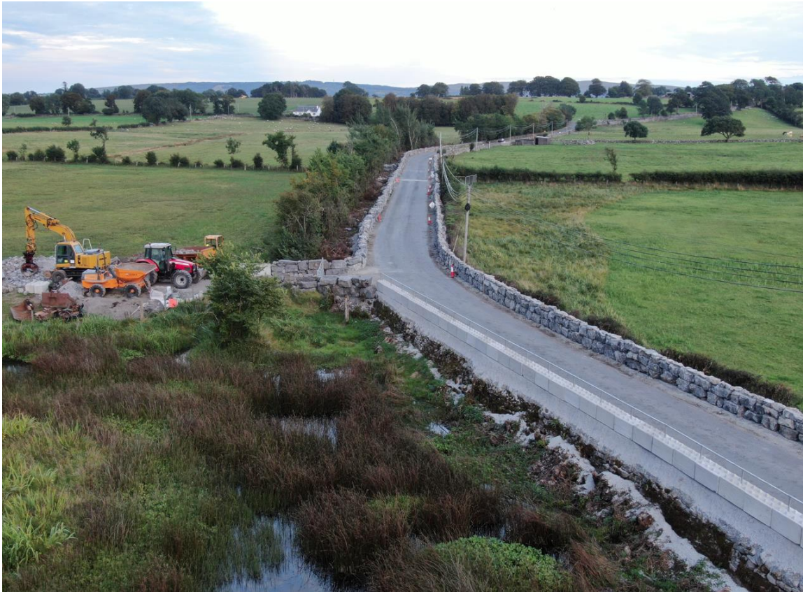
Works in progress - photo of the 'Pond', where crash resistant blocks and pedestrian rail have been installed to maintain the public visual amenity of the pond. Concrete reinforcement placed on top of existing 2m stone wall to support blocks. Rock armour walls substantially completed.
